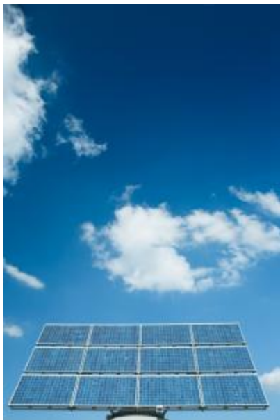
Figure 4: Solar PV panel
