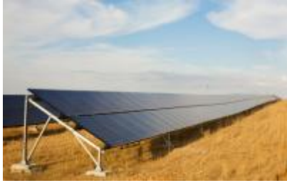
Figure 5: Ground mounted solar PV panels
