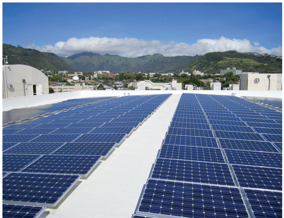
This 102 kW PV array in Mō'ili'ili, Hawaii, uses Sharp monocrystalline PV modules.
